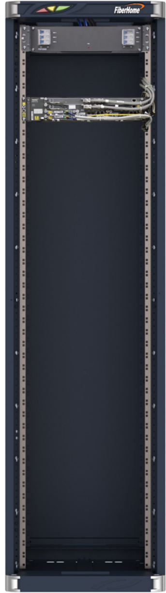
An MSAN Service Subrack
